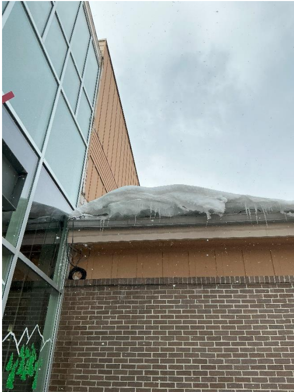
Photo 3: Ice Damming at Roof (Anderson Hallas Architects 2025)
