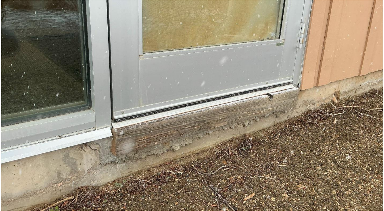
Photo 8: Wood sill at exterior door 118 (Anderson Hallas Architects 2025)
