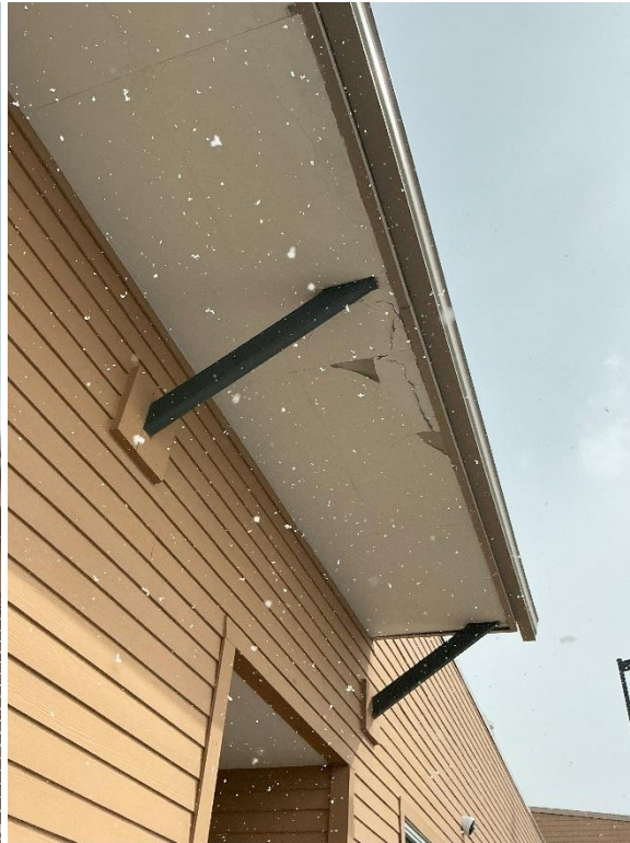
Photo 4: Damaged Soffit at Drive-thru/Staff Entry (Anderson Hallas Architects 2025)
