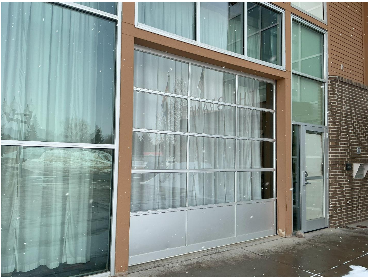
Photo 9: Overhead door at Community Room (Anderson Hallas Architects 2025)
