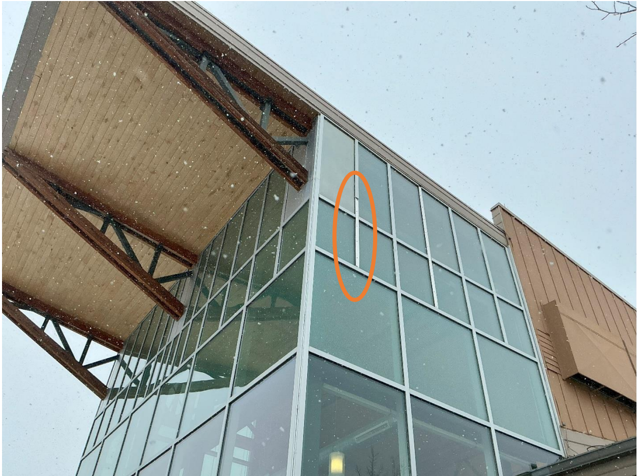
Photo 7: Curtainwall missing mullion caps (Anderson Hallas Architects 2025)
