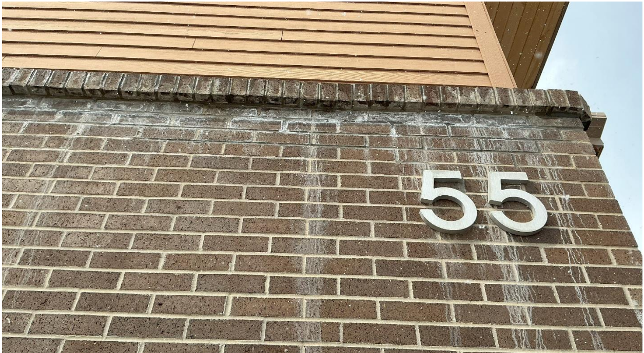
Photo 5: Efflorescence at rowlock ledge (Anderson Hallas Architects 2025)
